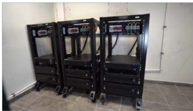
UPS EVER w data center
