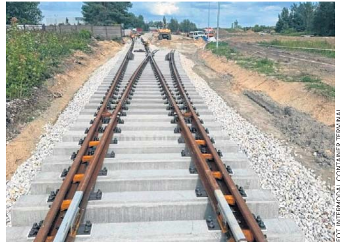
FOT. INTERMODAL CONTAINER TERMINAL
